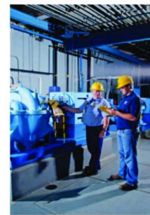
Water Treatment Equipment
